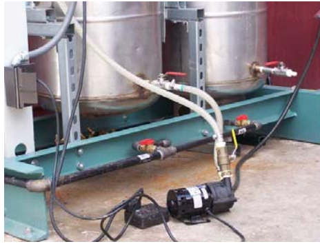
Magnetic drive pump circulating wort through the HERMS coil
