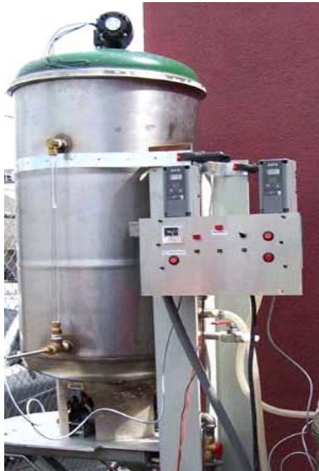
HLT with sight gauge and temp sensor Control Panel with Electronic Temp Controllers on top, pilot lights show status of pump and HLT burner
